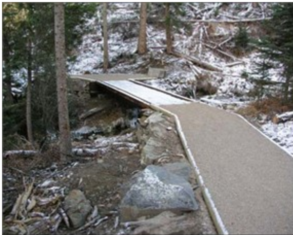
TC4 – Structures frequent and substantial. Substantial trail bridges are appropriate at water crossings.
